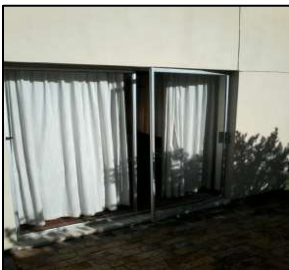
Figure 12: Sliding door pulled off rails by GOB5
